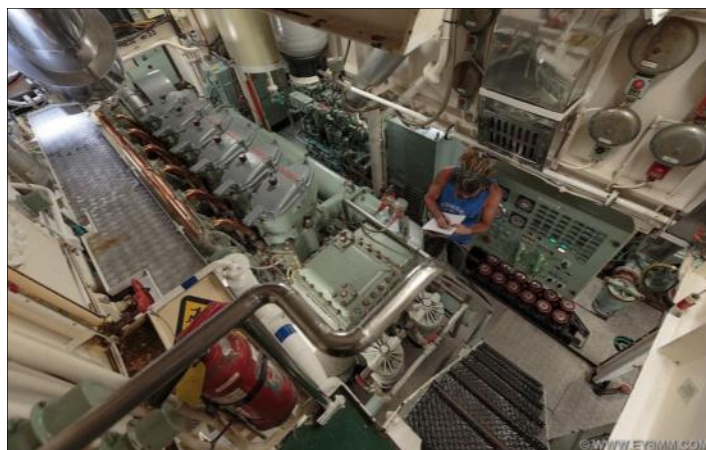
The Braveheart's engine room.
