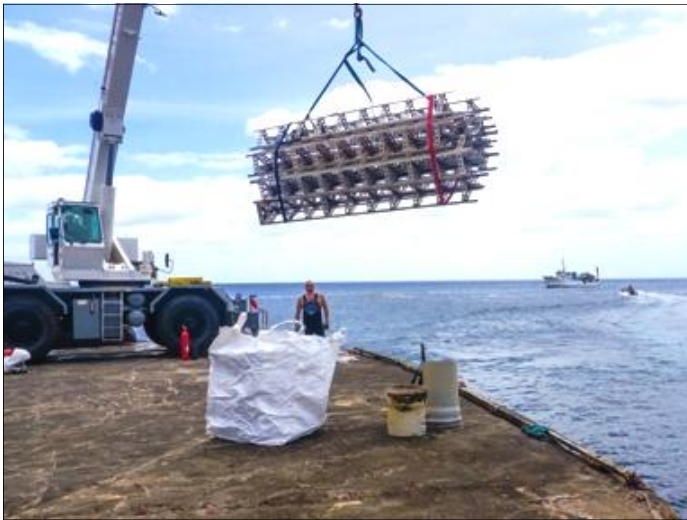
Tower sections being lifted ashore. These would support ten 3-element monoband Yagis.
