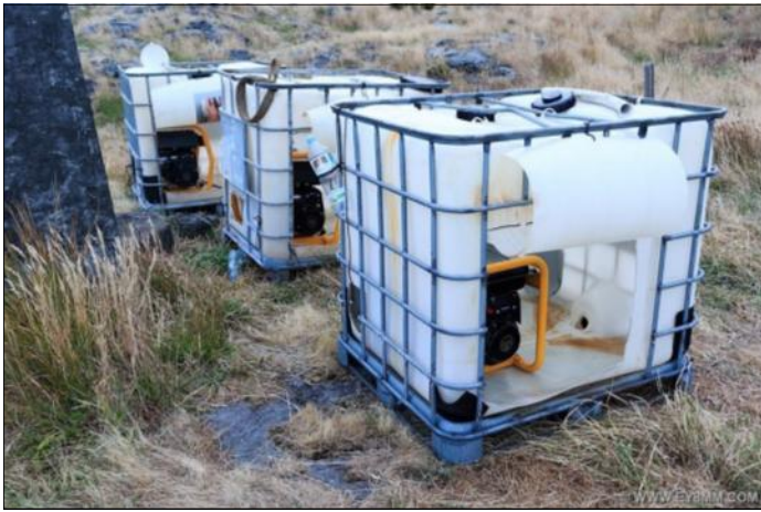
Generators run in special housings to prevent any oil or gas spills.
